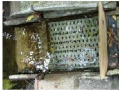
Perforated galvanized cable tray intake
